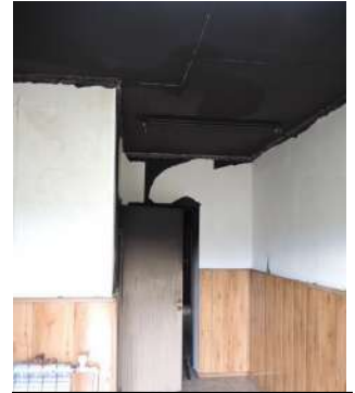
Damaged walls & ceiling in the remaining building
